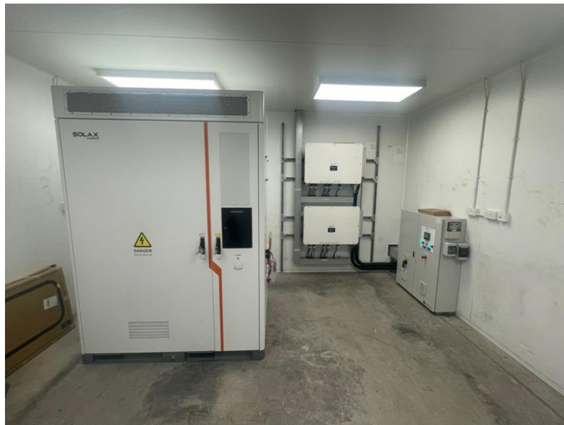
ASG AMF's battery storage (shown during installation) is housed in the factory within a dedicated module.
