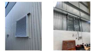
AIR INTAKE LOUVERES w/ DAMPERS
